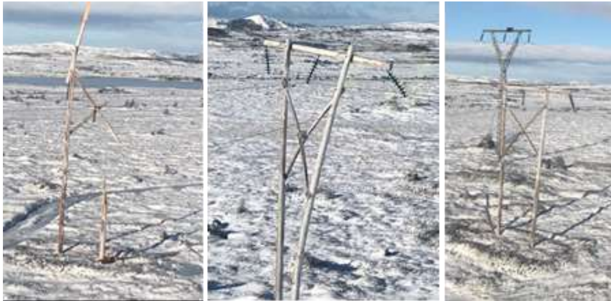
Figure 6: TL219 Structure Failures and Mechanical Bending
