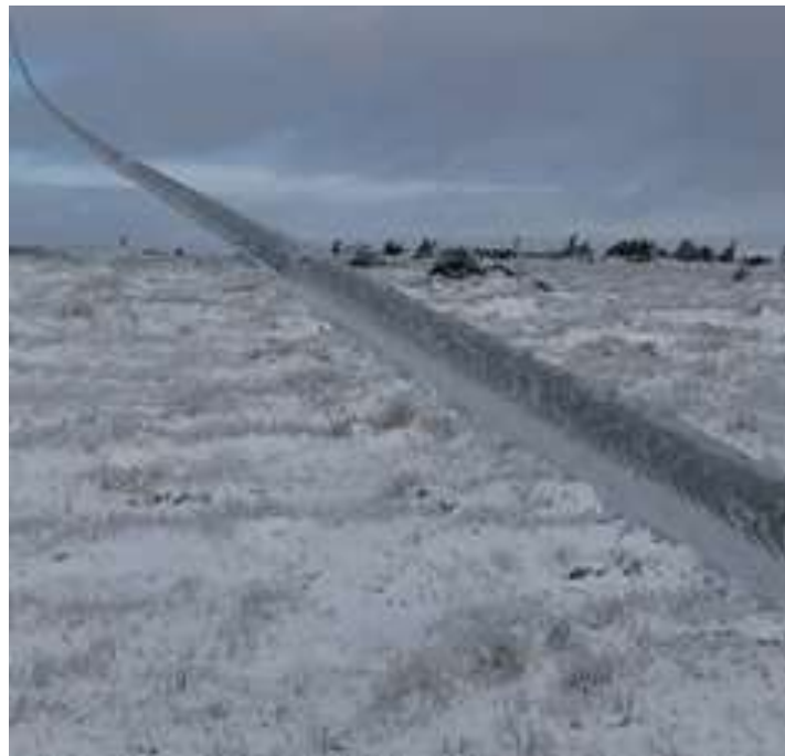
Figure 2: Ice Accumulation on TL219 Conductor
