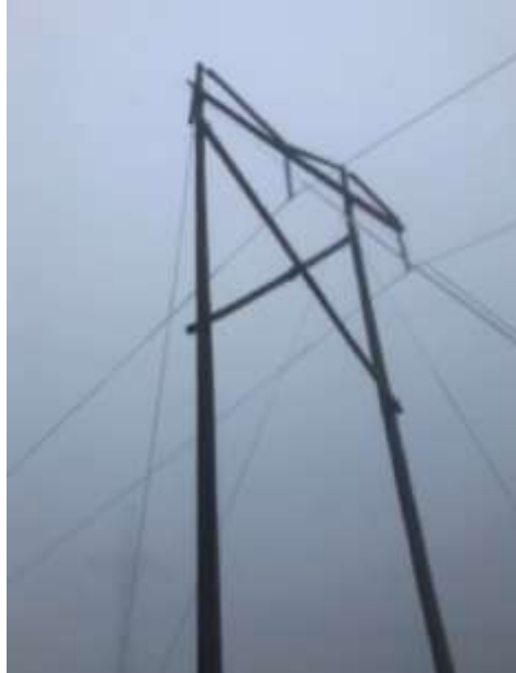
Figure 9: Broken Crossarm on TL203 – Structure 77
